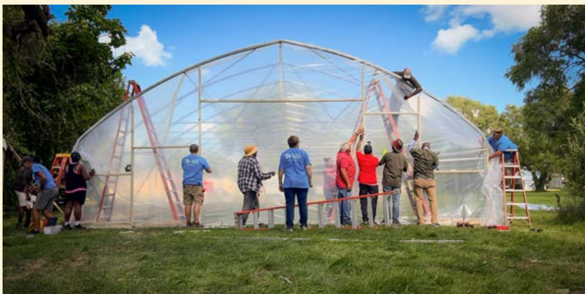
Volunteers work with local organizations and USDA NRCS staff to build a high tunnel at a church in Waterloo, Iowa. The church is in a neighborhood considered to be a food desert.
